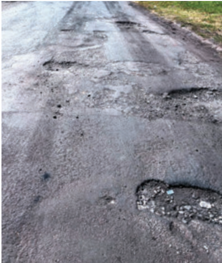
Before – Dawes Street was filled with potholes which posed a threat to motorists.
