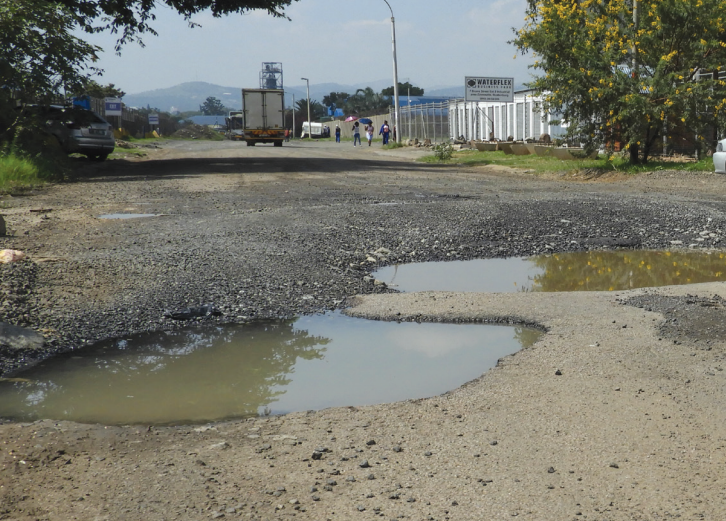
Commuters now have to take the road less travelled: literally driving next to the road to avoid damaging the vehicles.
