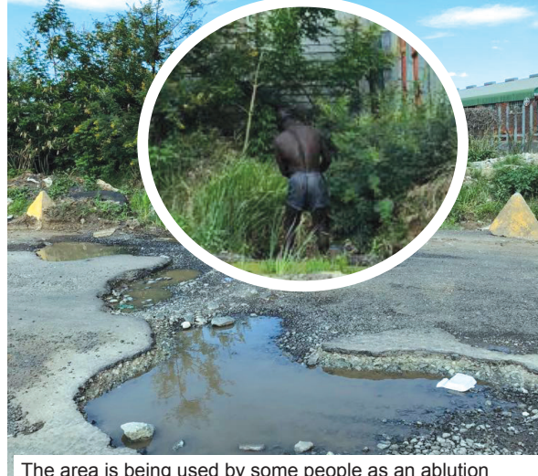
The area is being used by some people as an ablution facility, people are often seen washing themselves in this water, and this could become a major health hazard.
